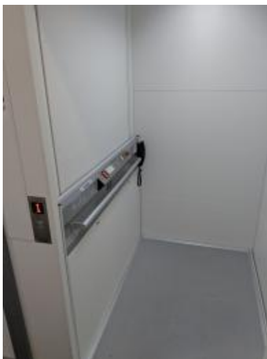
Inside the lift.
